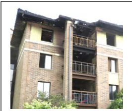
162 Units – 06/01/26 Fire. Glendale, WI
